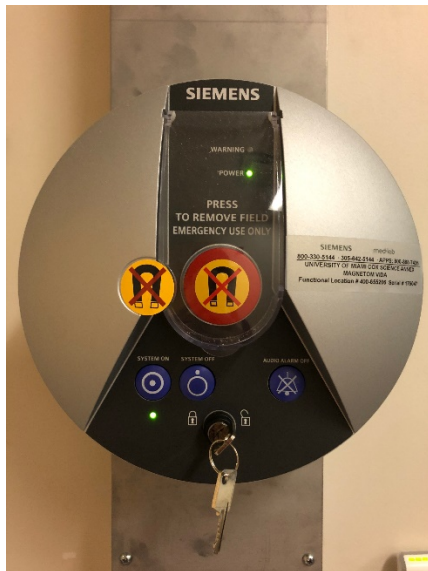
Figure 4. Quench button in the control room.
