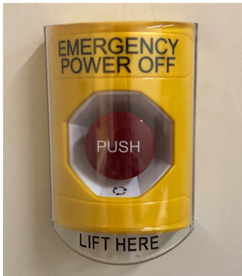
Figure 5. Emergency Off Button in the control room.
