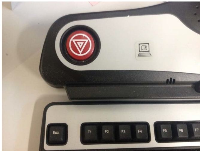
Figure 5. Emergency Off Button in the control room.
