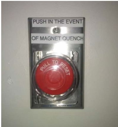
Figure 4. Quench button in the control room.
